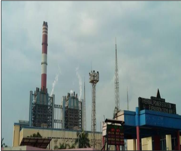
Coal Handling Plant
